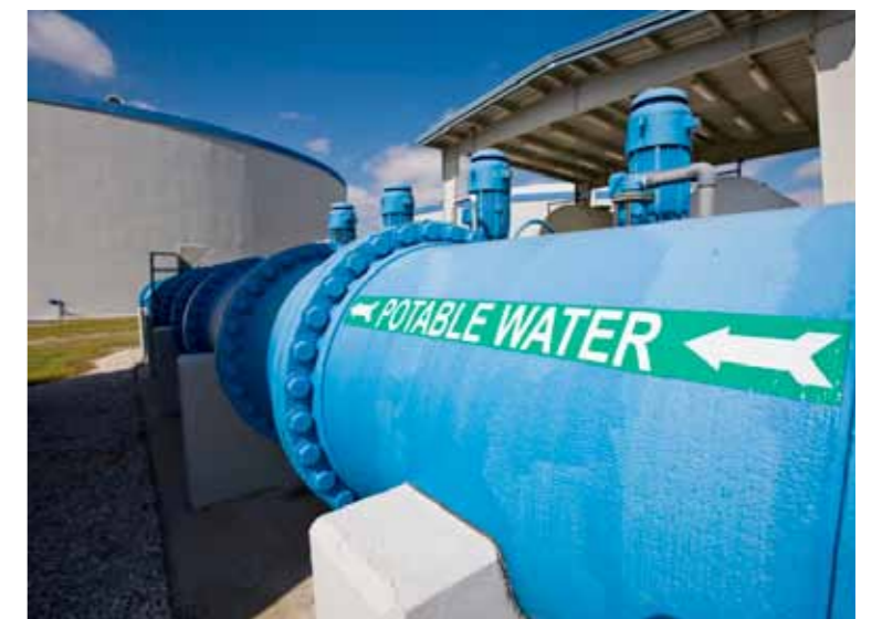
FIGURE 67 - DESALINATION PLANT: SERVICING ESPERANCE LOCALLY AND THE BROADER GOLDFIELDS - ESPERANCE REGION
