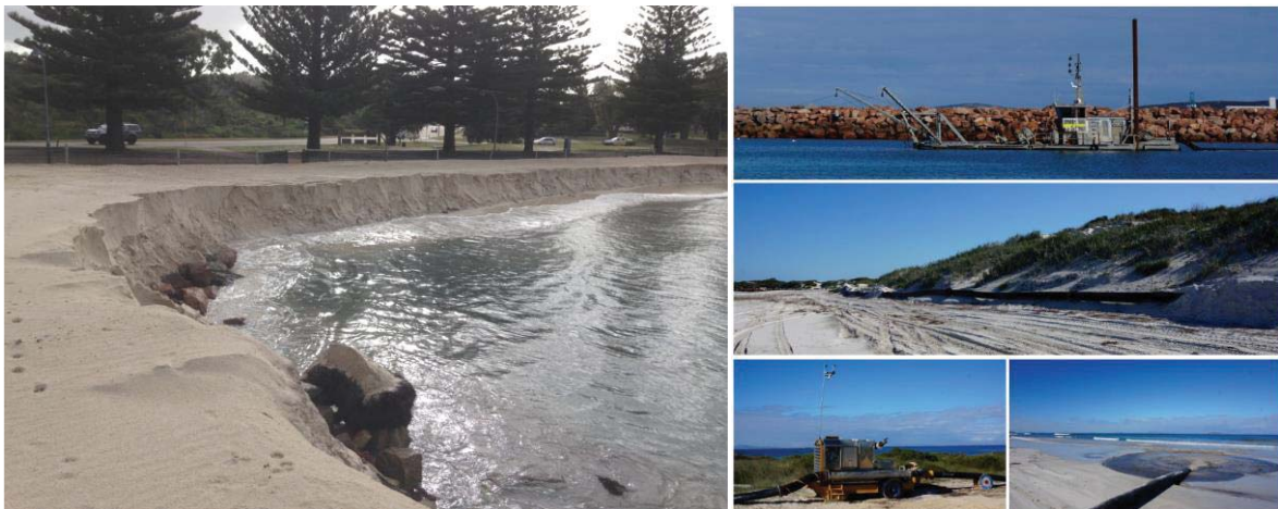
Figure 1.1: Beach nourishment at Castletown Beach in coordination with the DoT's Bandy Creek Boat Harbour dredging
