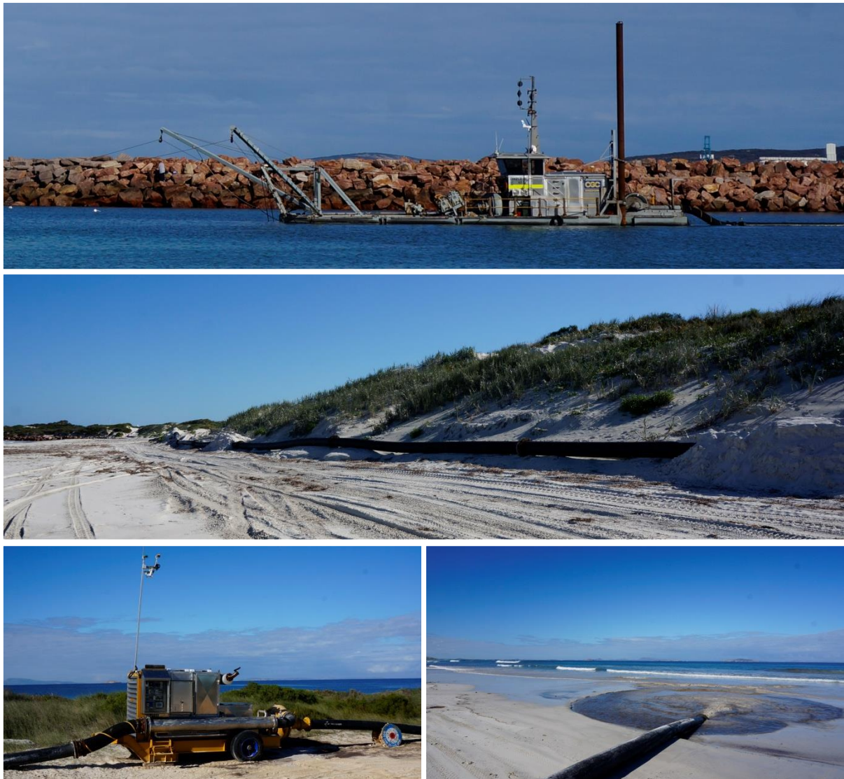
Figure 3-6: Illustration of dredging and beach disposal at Bandy Creek Boat Harbour (dredge, slurry pipeline, booster pump and discharge pipeline).
