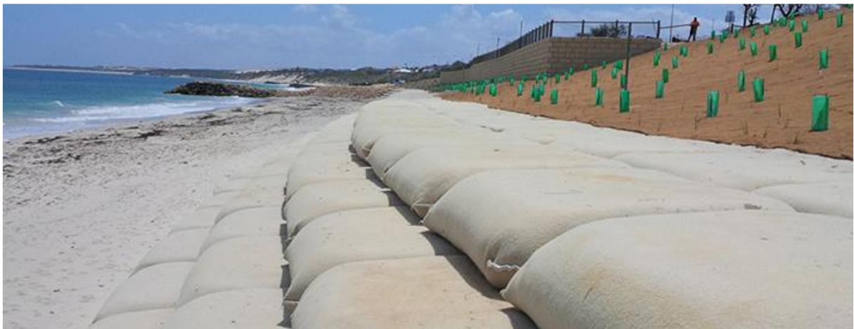
Figure 3-8: Illustration of seawall options – top: Esperance Foreshore, WA (rubble-mound seawall); bottom: Quinn’s Beach - Wanneroo, WA (geotextile seawall, photo credit: http://www.tessilbrenta.com ).
