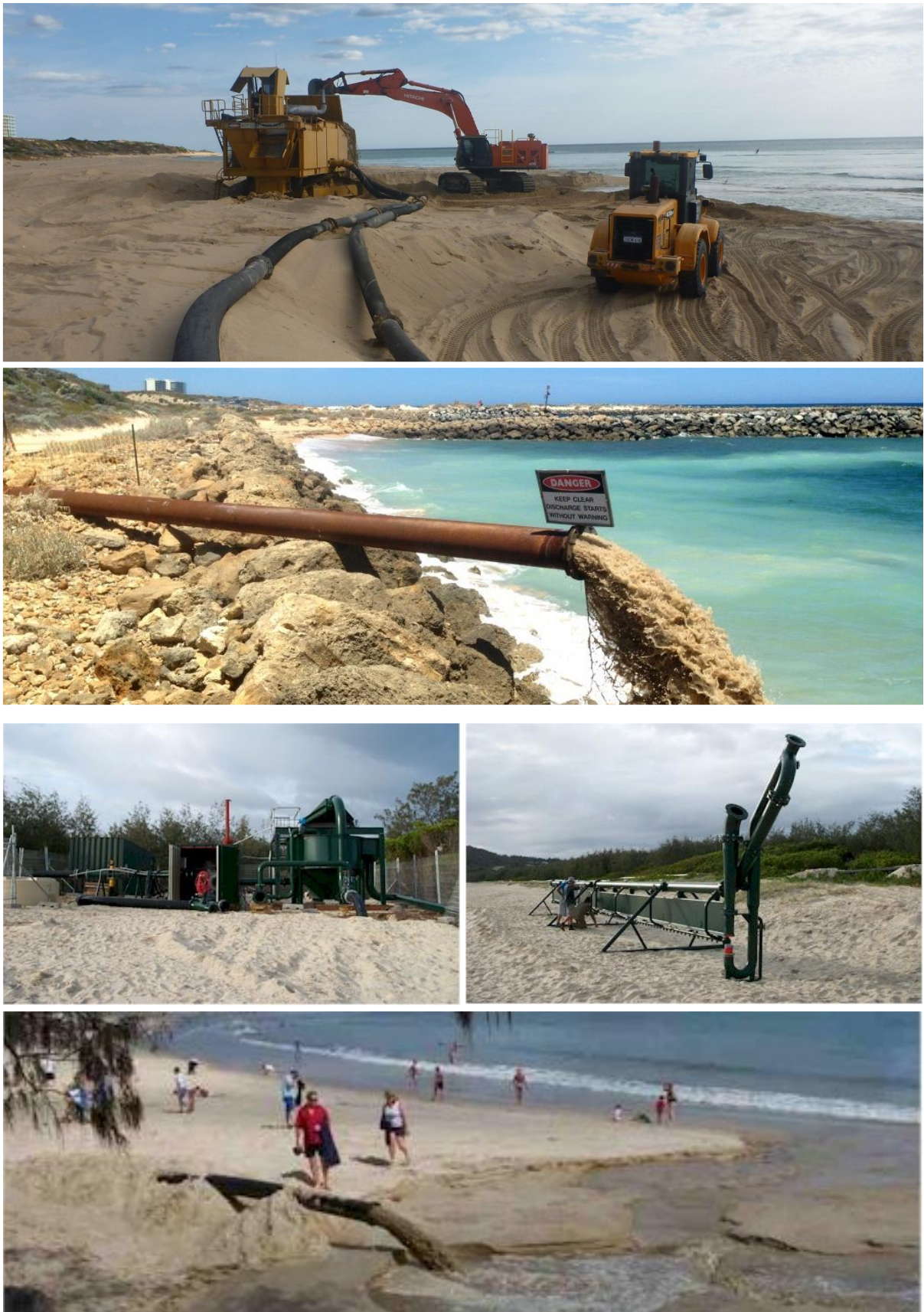
Figure 3-3: Illustration of mobile sand back-passing - Top two: Dawesville, WA (Excavator, mobile slurry trap and discharge pipeline). Bottom three: Noosa, QLD (Pump station, sand shifter and discharge pipeline).
