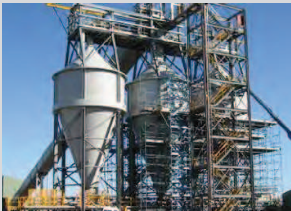
Roche Minerals – 2000t Silo
