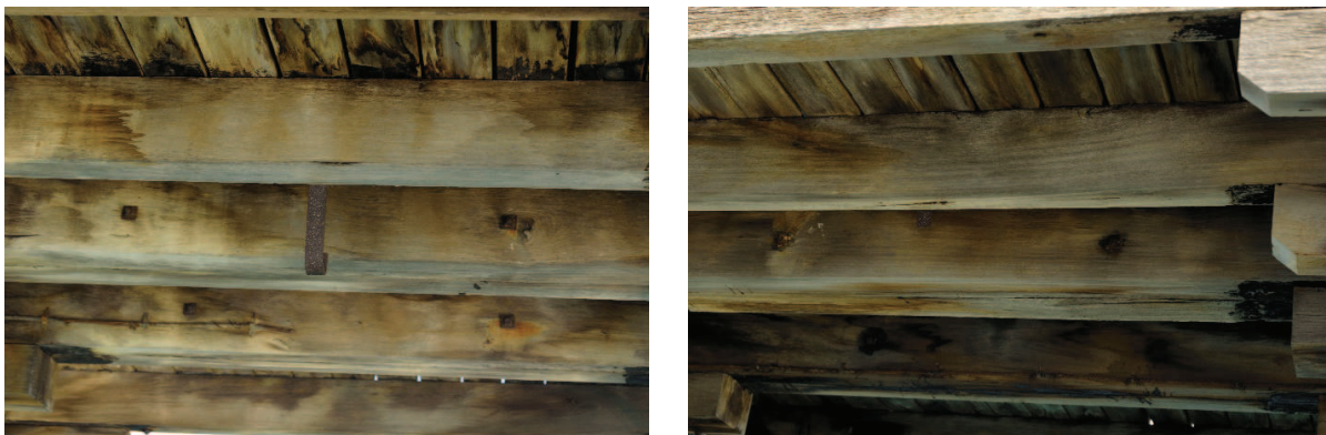
Examples of typical internal stringers is relatively sound condition
