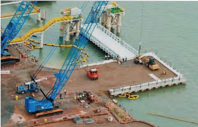
GLNG – RG Tanna - RoRo Facility during construction Superlift Manitowoc crane installing the linkspan bridge (110t) as a single crane lift
