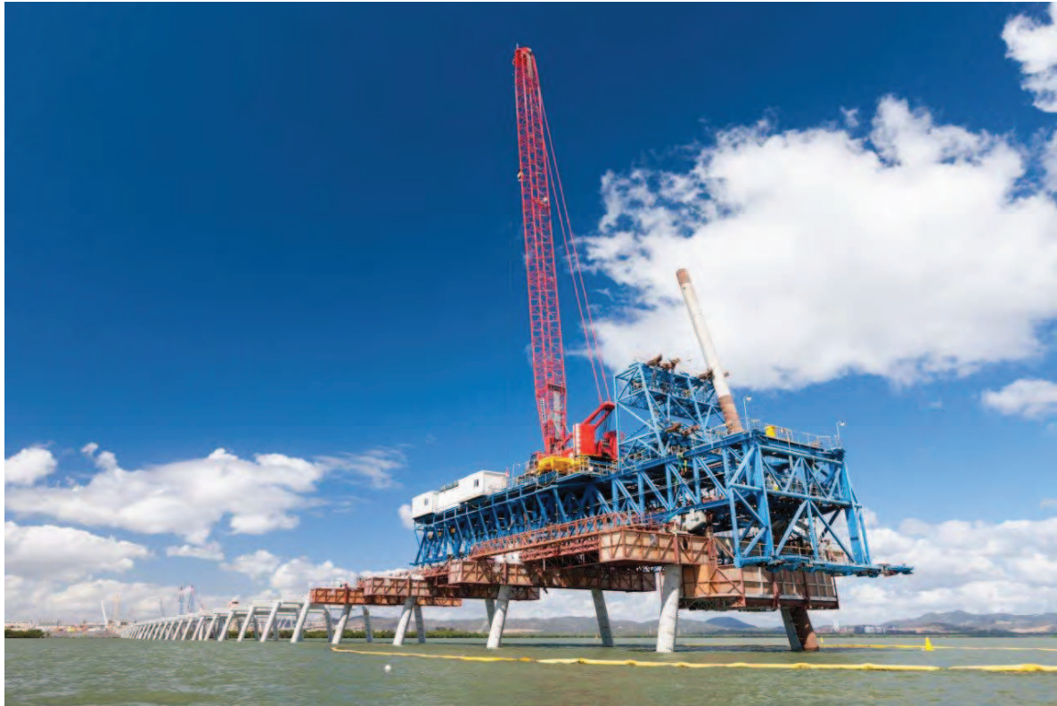
Wiggins Island Jetty Traveller
