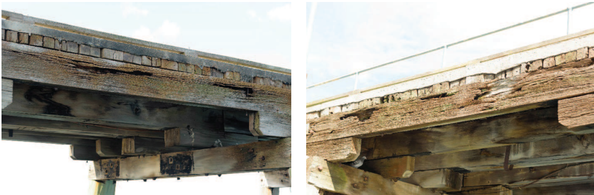
Examples of typical external stringers that require replacement or structural augmentation
