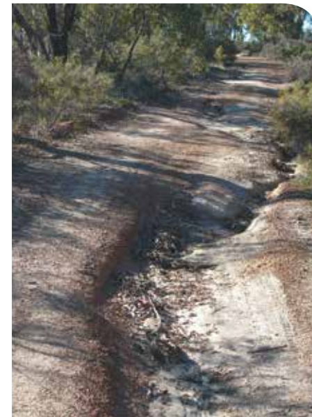
Above: Water erosion on a fire-break without adequate erosion-prevention measures.
