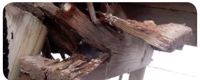
Failure of Half Caps
