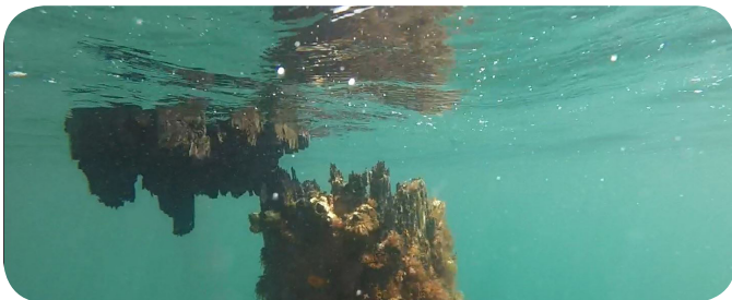
Failure of Piers
