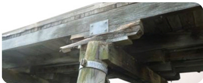
Crushing and Failure of Corbels
