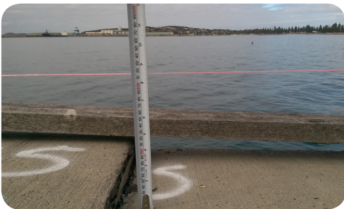
Sag in deck planking at pile 95s
