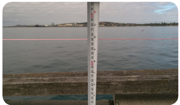
Sag in deck planking at pile 94s
