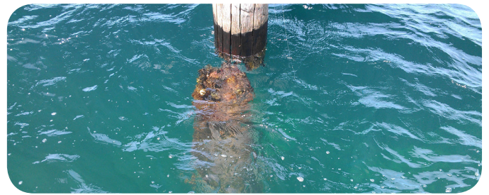
Failure of Piers
