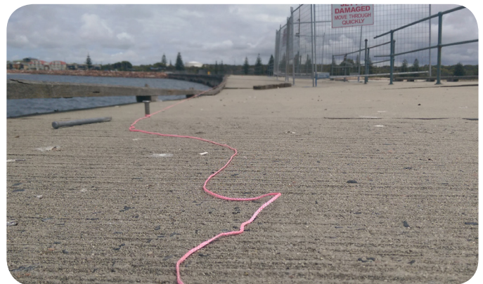
Sag in deck planking
